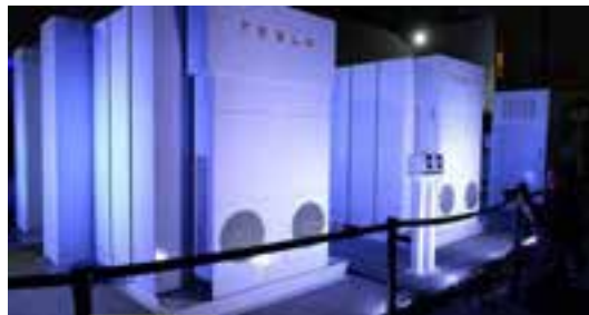
image of a Tesla PowerPack . Tesla built and installed the world's largest lithium-ion battery in Hornsdale, South Australia, using Tesla PowerPack batteries. Since then, the facility saved nearly $40 million in electricity costs its first year alone and helped stabilize the region's unreliable electric grid.
