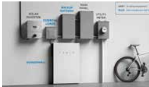
image of a Tesla PowerWall in the basement of a homeowner. Note the Tesla PowerWall on the basement floor and its connection to the "SOLAR INVERTER" which sends solar energy to be saved in the PowerWall
