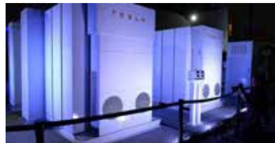
image of a Tesla PowerPack . Tesla built and installed the world's largest lithium-ion battery in Hornsdale, South Australia, using Tesla PowerPack batteries. Since then, the facility saved nearly $40 million in electricity costs its first year alone and helped stabilize the region's unreliable electric grid.
