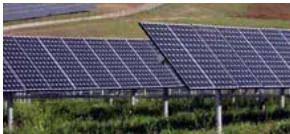
solar panels on a solar farm in the European country of Portugal
