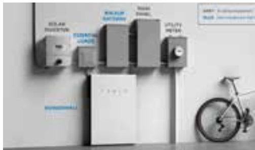
image of a Tesla PowerWall in the basement of a homeowner. Note the Tesla PowerWall on the basement floor and its connection to the " SOLAR INVERTER " which sends solar energy to be saved in the PowerWall
