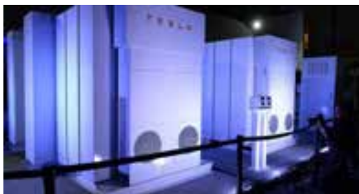
image of a Tesla PowerPack . Tesla built and installed the world's largest lithium-ion battery in Hornsdale, South Australia, using Tesla PowerPack batteries. Since then, the facility saved nearly $40 million in electricity costs its first year alone and helped stabilize the region's unreliable electric grid.
