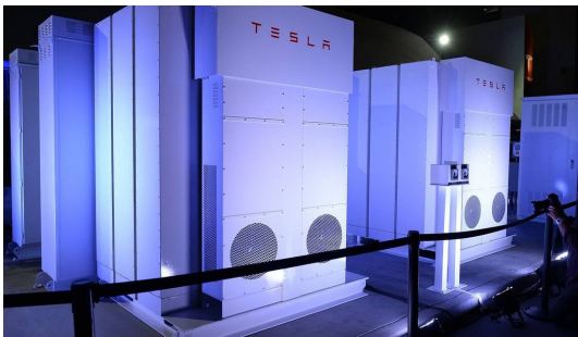
image of a Tesla PowerPack. Tesla built and installed the world's largest lithium-ion battery in Hornsdale, South Australia, using Tesla PowerPack batteries. Since then, the facility saved nearly $40 million in electricity costs its first year alone and helped stabilize the region's unreliable electric grid.
